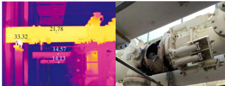
Figure 6. Local overheating caused by poor contact, current overload, etc.
